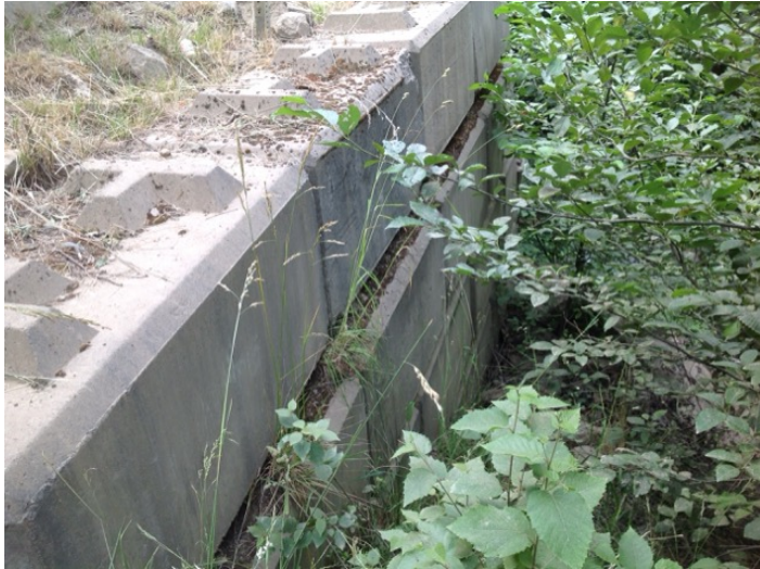
right downstream wall battered
